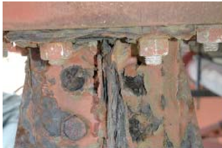
Rusting on the Bridge
